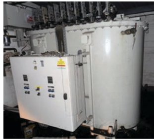
Bernard and Bonnefond Varivolt Transformer
